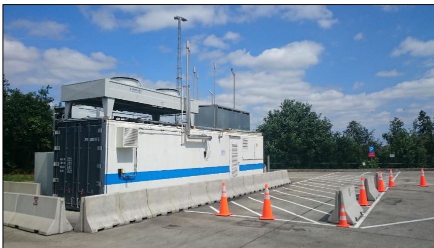
Foto 3: PEM electrolyser and fuel cell are installed (August 2015)
